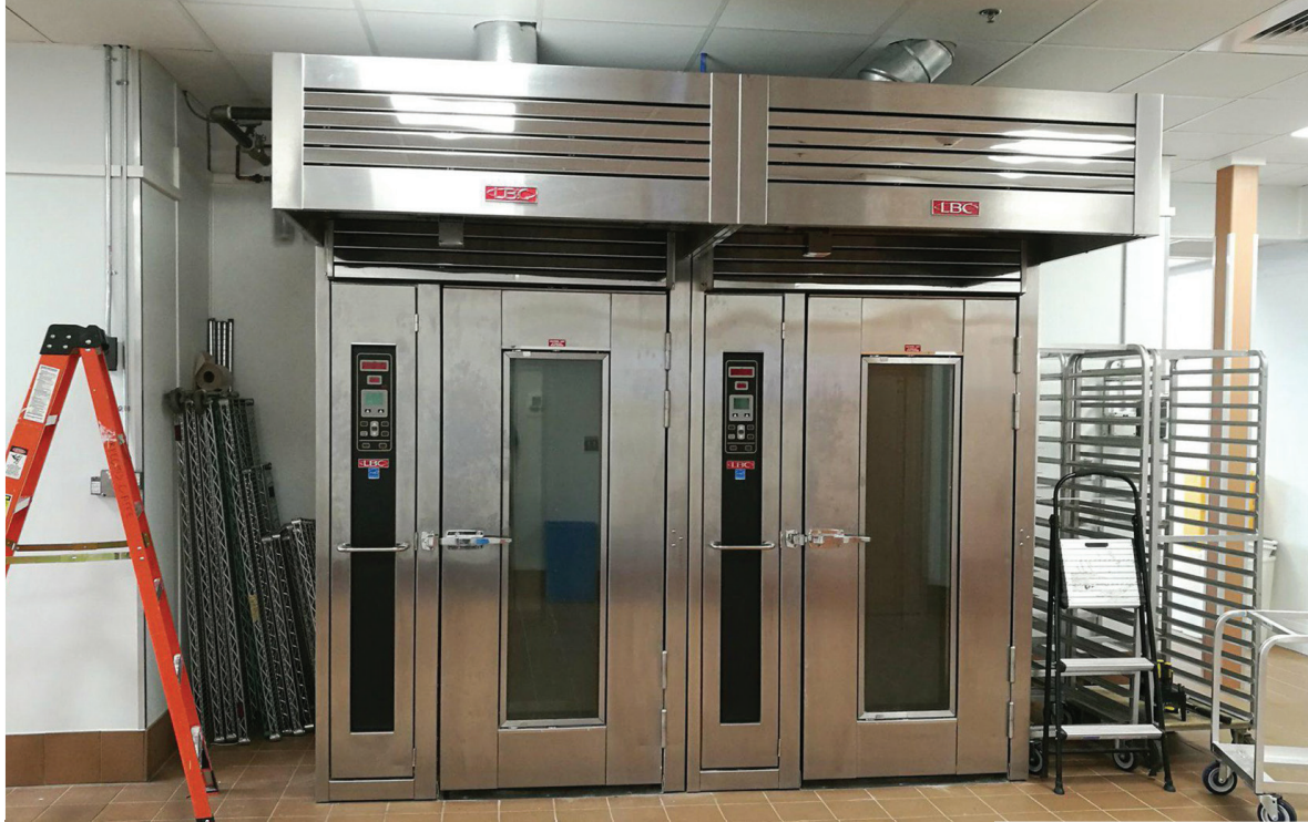
CRN Plumbing doesn't just work in residences—its expertise extends to commercial projects as well.
