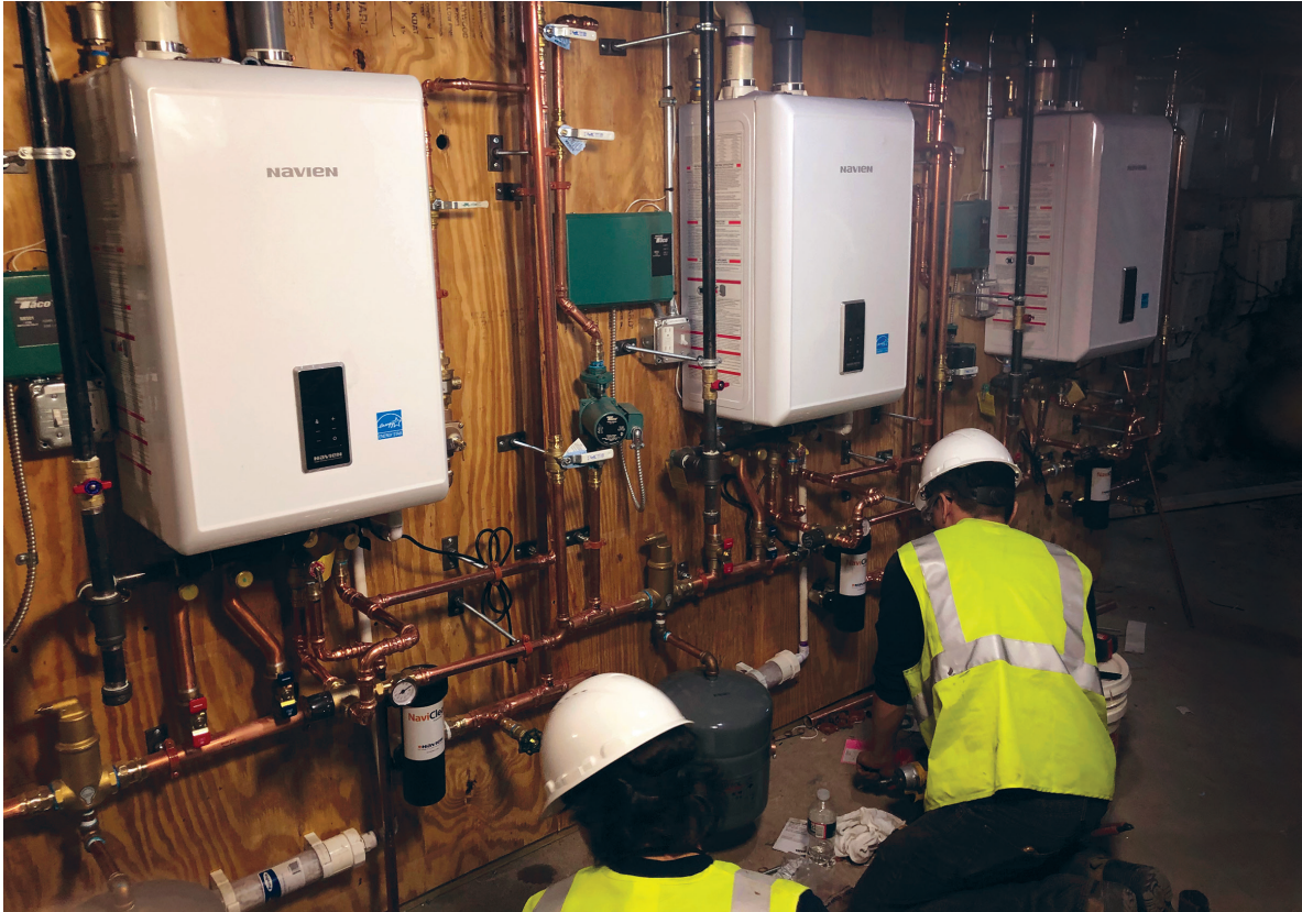
The CRN Plumbing team helped the victims of the Merrimack Valley gas explosions by repairing and replacing high-efficiency boilers, furnaces and water heaters at residential properties.
